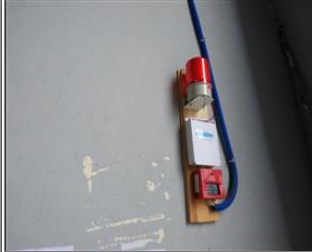
Photo of the inside of the main production hall Fire alarm.jpg
