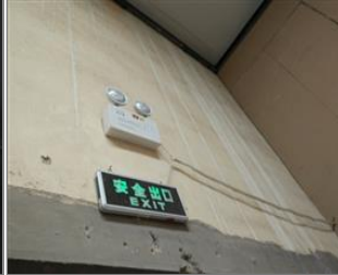
Photo of the inside of the main production hall Safety exit sign and emergency light.jpg
