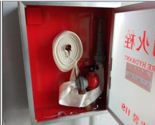
Photo of the inside of the main production hall Fire hydrant.jpg
