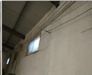
Photo of non-conformity Electrical wires were not sleeved with nonflammable tube in warehouse.jpg
