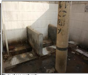
Photo of non-conformity The sanitary condition of toilets was poor no private door was installed in the toilet and no basic necessities such as toilet paper and soap were provided in the toilet.jpg
