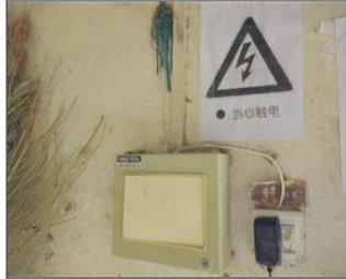
Photo of the inside of the main production hall Electrical box with warning sign.jpg
