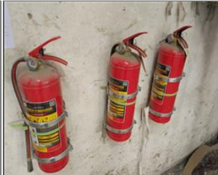
Photo of the inside of the main production hall Fire extinguishers.jpg
