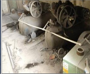
Photo of non-conformity No belt guard was equipped on the air compressors.jpg
